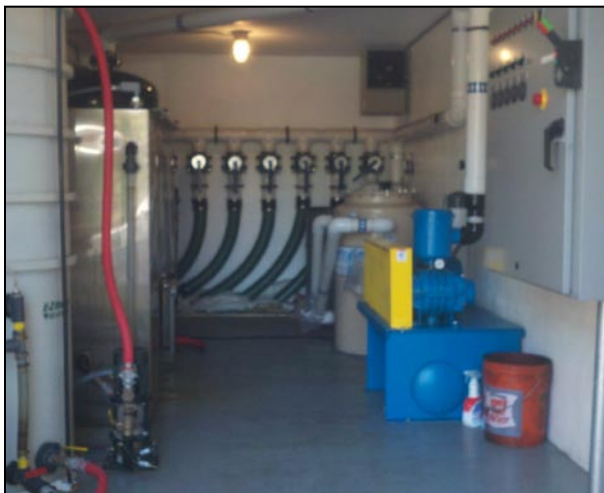
DPE REMEDIATION SYSTEM INTERIOR VIEW
