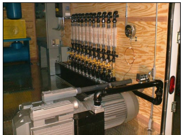
SVE/ AIR SPARGE REMEDIATION SYSTEM INTERIOR VIEW
