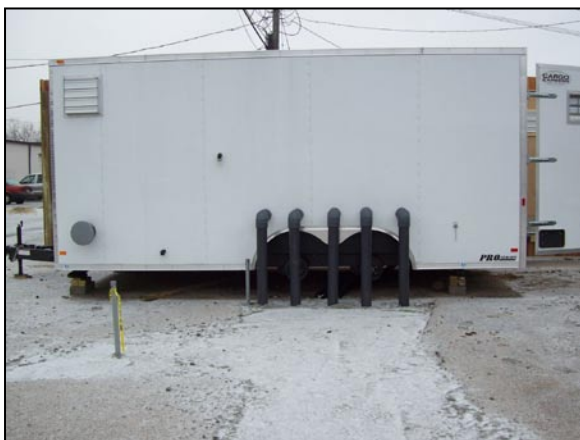
SVE/ AIR SPARGE REMEDIATION SYSTEM EXTERIOR VIEW
