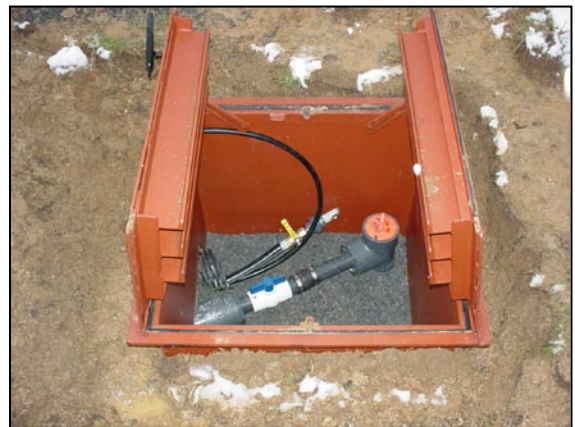
DPE WELL-HEAD ASSEMBLY, HOUSED WITHIN ACCESS VAULT.
