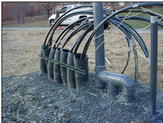
DPE SYSTEM CONNECTIONS: VACUUM, GROUND WATER INFLUENT, AND PNEUMATIC PUMP AIR SUPPLY.
