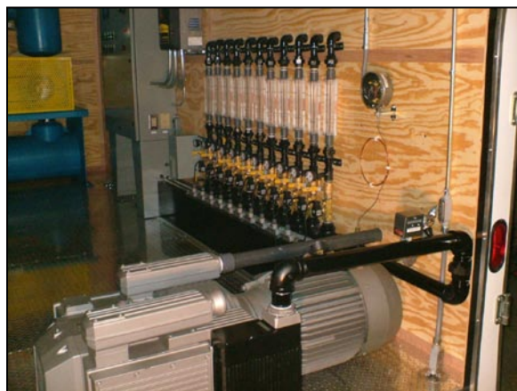
SVE/ AIR SPARGE REMEDIATION SYSTEM INTERIOR VIEW
