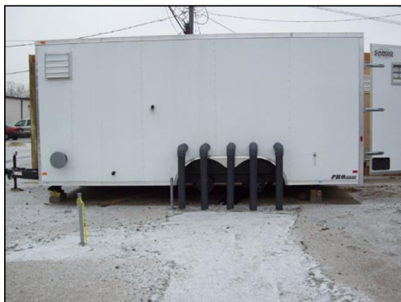
SVE/ AIR SPARGE REMEDIATION SYSTEM EXTERIOR VIEW
