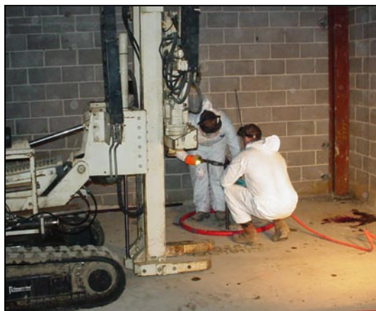
DIRECT PUSH INJECTION POINT WITHIN BUILDING
